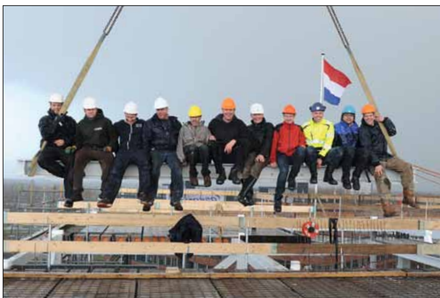
And then, the last beams were put in place. At the topping out ceremony, builders and CHDR people enjoyed a good view and a fresh splash of rain. Candidate compounds which proved effective against acrophobia contributed to the festive atmosphere.
